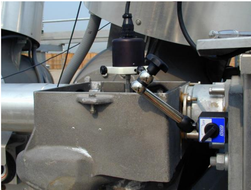
Rotary Transducer on Alstom HE 1014 Circuit Breaker
